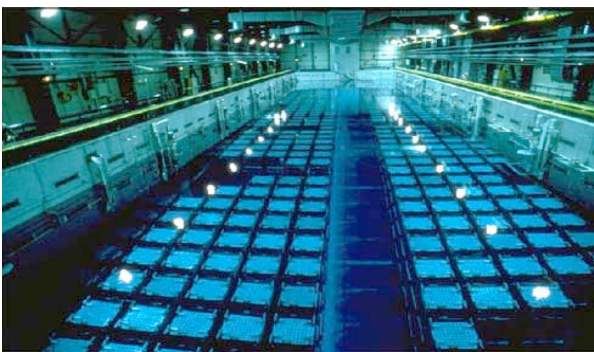
Figure 1 – Main spent fuel pool in La Hague
