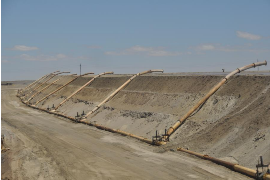
Slurry Pipelines on Tailings Dam, Rössing Mine, Namibia.
